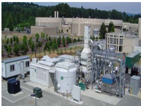
Fig. 3. King County DFC1500 fuel cell power plant: the plant operates on digester gas and on natural gas when digester gas is not available.
